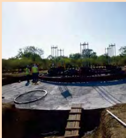
Ventika Wind Farm
